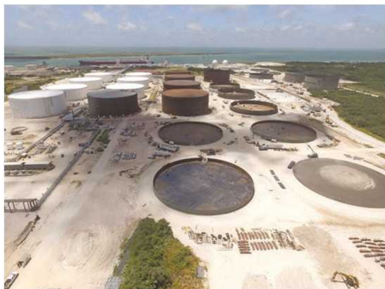
Matrix is providing EPC services on 14 aboveground storage tanks and related balance of plant, adding 7 million barrels of storage capacity at the Moda Ingleside Energy Center.
