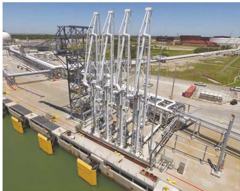
New Berth 2A installation by Matrix allows for mooring of very large crude carriers and provides improved loading capabilities of up to 80,000 barrels per hour with 99.9-percent VOC emissions recovery.
