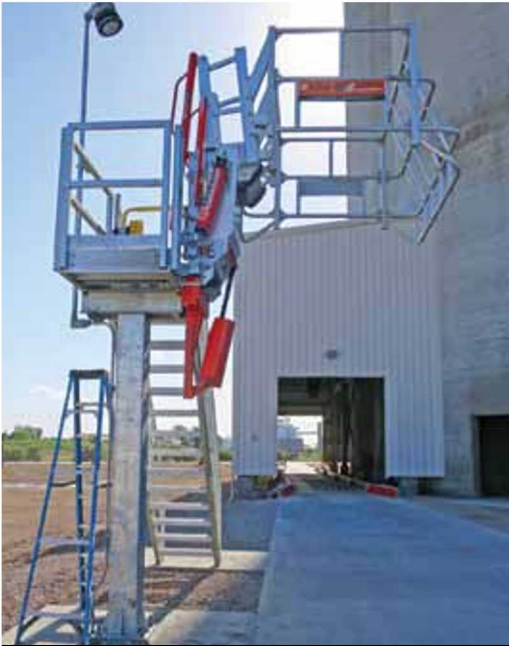
New fourth truck load-out lane at the Houston Cement facility, Port of Houston, USA
